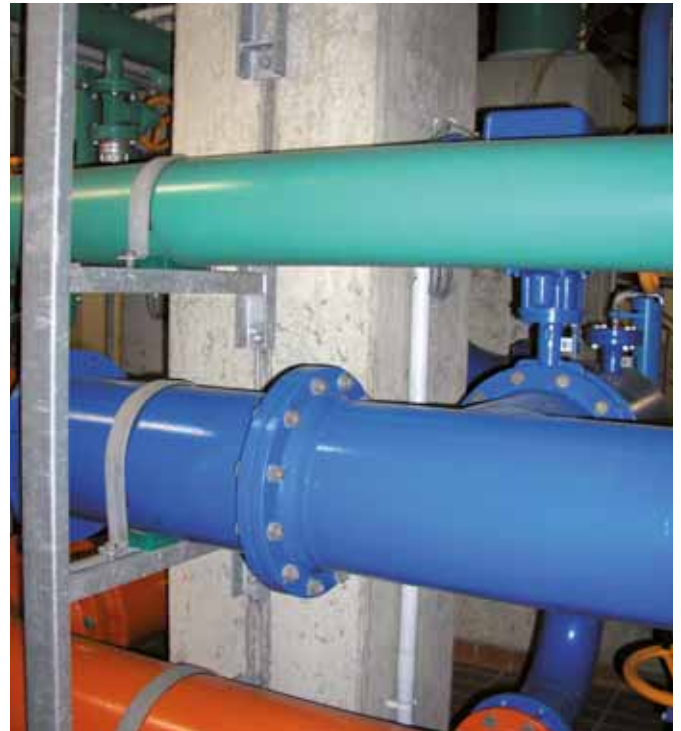
Pipe support fixed to vertical cast-in serrated channel
