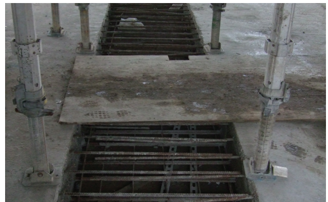
Pour Strips restrict site access, create hazards and delay progress on site.
